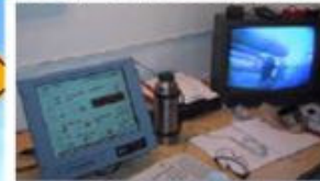
View of the control room
